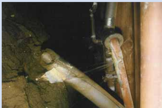
Buildings that aren't occupied regularly may have small problems such as slowly leaking pipes that go undetected for years.
