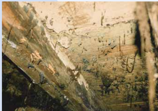
A small amount of mold visible to building occupants can very likely be the sign of bigger problems.
